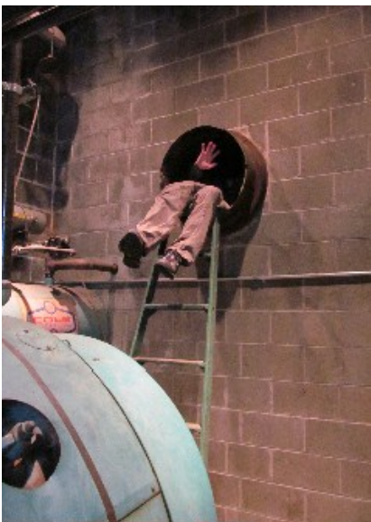
Larry Schwitters goes the distance to install temperature loggers in the Monroe School District Administration Building chimney to monitor Vaux Swift roosting conditions
