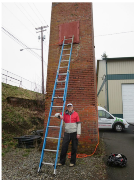
Larry Schwitters working on closing an opening in a potential Swift migratory chimney in Chehalis. Feb 2016
