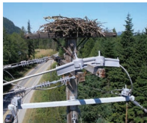
Insulator cover near nest
